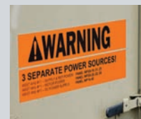
Equipment and panel labeling
