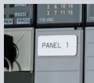
Control panel labels
