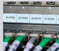
Patch panel and terminal block ID
