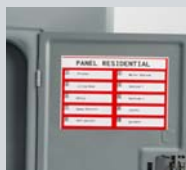
Residential panel labeling
