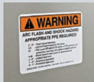
Arc flash labeling
