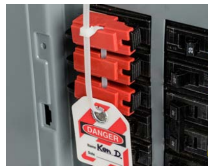
120V breaker lockout devices fit on breakers next to each other, enabling multiple tagouts at one time
