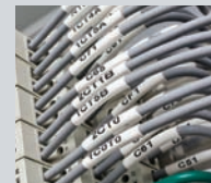
Wire and cable labels
