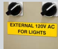
Equipment and panel labeling
