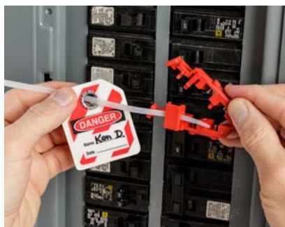
Save time by "pre-loading" your tag and cable tie before walking to the energy point
